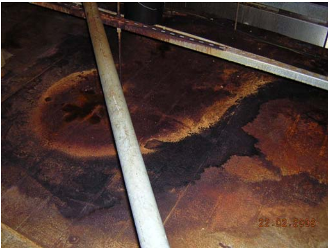
Typical abuse to ceiling panels from leaks and spills
